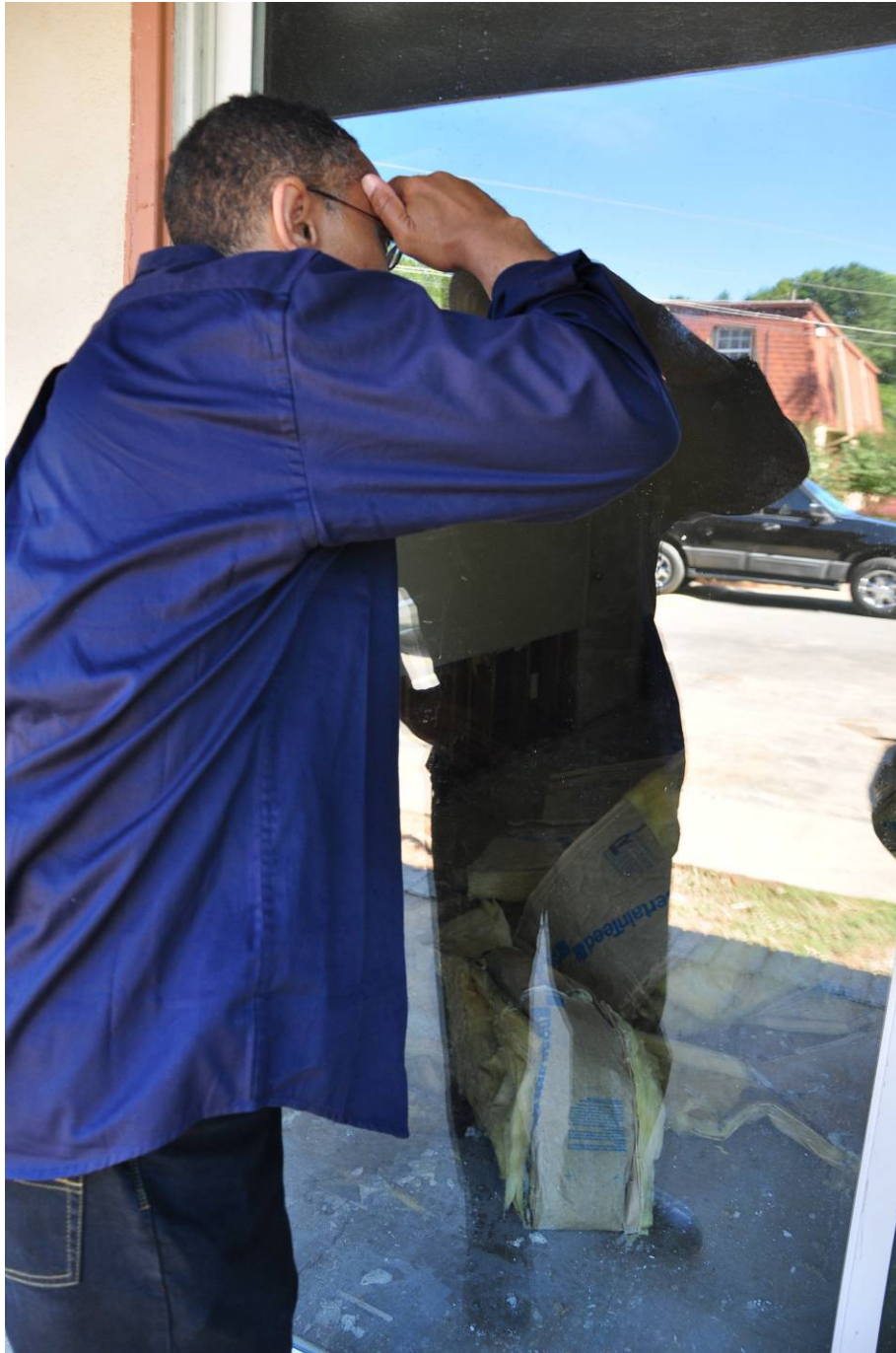
CEO Ellis inspecting flood damaged apartment at Casa Mia Heights
